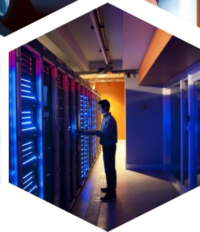
Data center cooling
